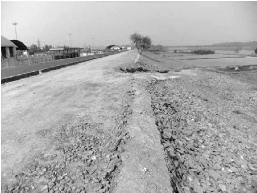
Figure 11.5 DTC Bus Depot and new embankment (Photo by Alexander Follmann, taken on 7 November 2011)
