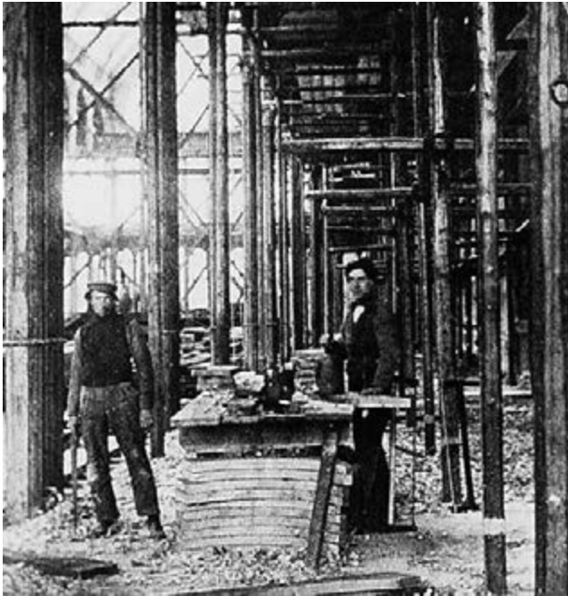
Figure 3.1 Carpenters at the construction of the Paleis voor Volksvlijt (Palace of People's Industry), Amsterdam, c. 1862
