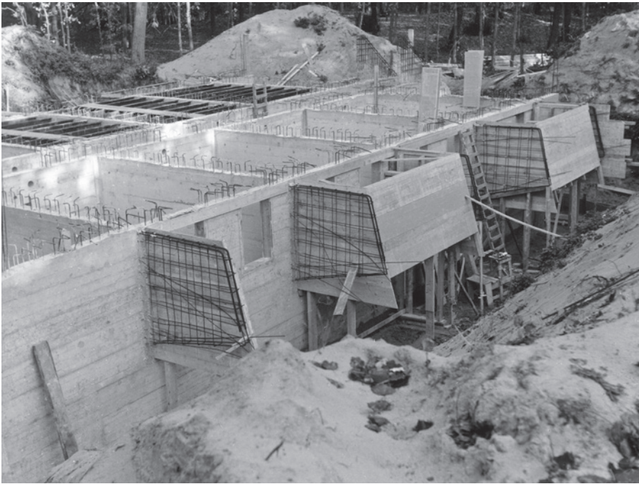
5: The nitrate vaults at Overveen under construction (Collection EYE Film Institute Netherlands)
