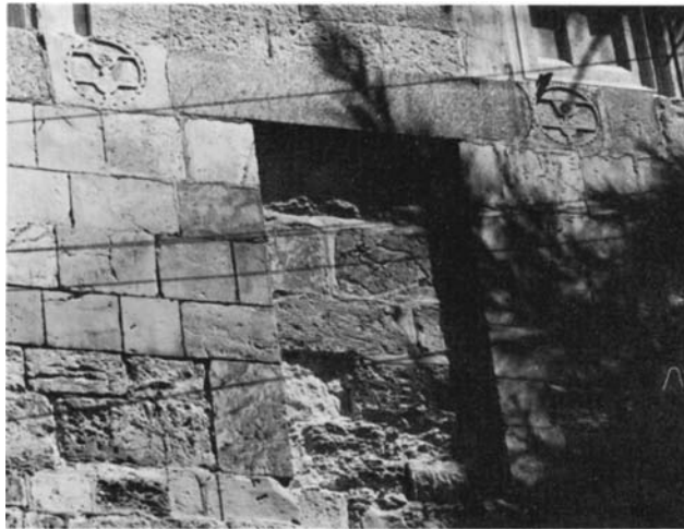
Plate 51.2 Blocked door in Haram façade, showing blazons on either side of lintel
