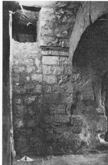
Plate 43.4 Blocked staircase to south-east mezzanine and roof with breach 'b' to right
