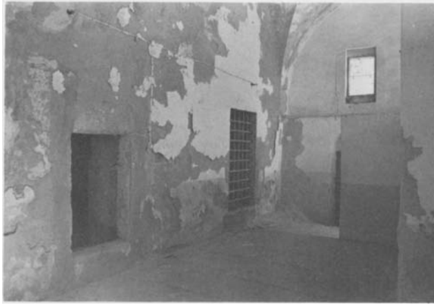
Plate 21.5 Door into ṭwān and window to 'tomb chamber', seen from under Ḥaram portico looking north-east
