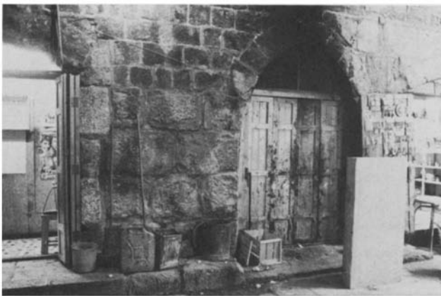
Plate 24.2 Junction at bays 16 and 17, south side, showing entrance to service area of Ḥammām al-Shifā'
