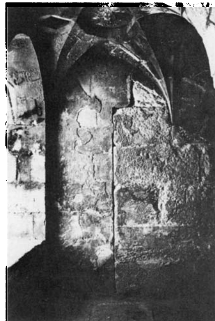
Plate 63.10 Break in masonry bond on south side of staircase
